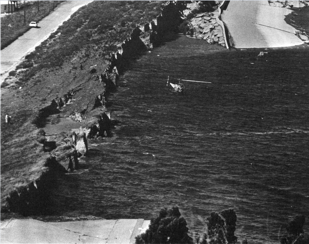
Lower Van Norman Dam: earthquake damage to this earth-fill dam posed a major flood threat. Photo credit: Los Angeles Times. Source: CALIFORNIA GEOLOGY magazine, April-May 1971.
